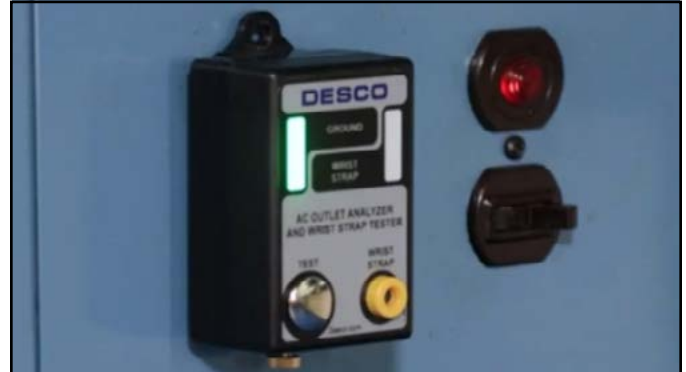
Figure 5. Verifying a properly wired AC outlet
