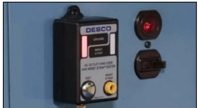
Figure 6. Verifying a properly wired AC outlet
