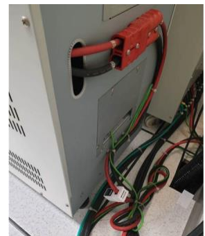
UPS Power Consumption Monitoring
